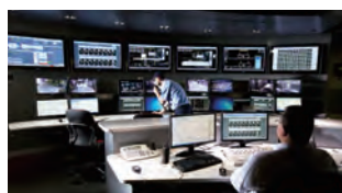
Command and control center
